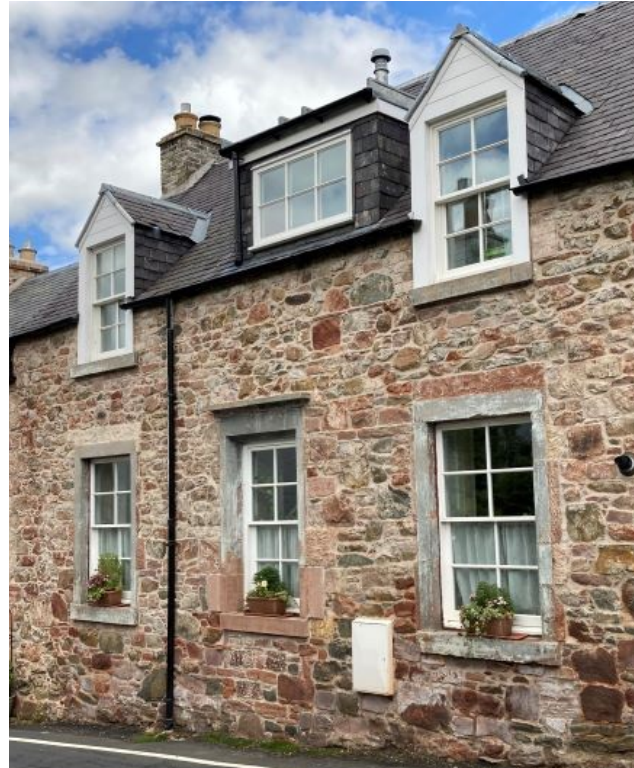
Fig. 56 To the left and right, traditionally-scaled and detailed dormers align with the windows below. This format could be followed. To the centre, a later box dormer of non-traditional design and poorly-aligned with windows below. This format would not be acceptable where visible in the streetscene.
